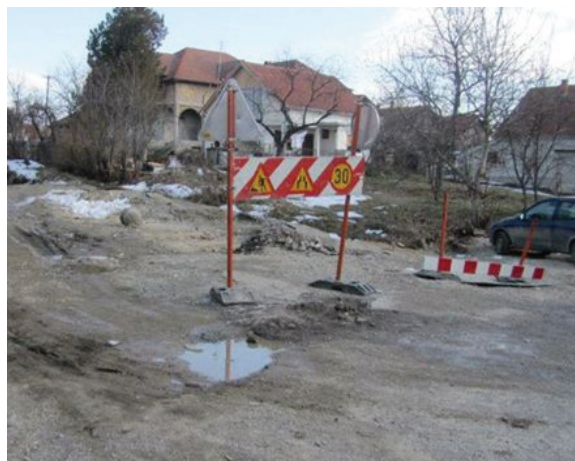
Figure 1. An example of poor regulation and direction of traffic in the roadwork zone
