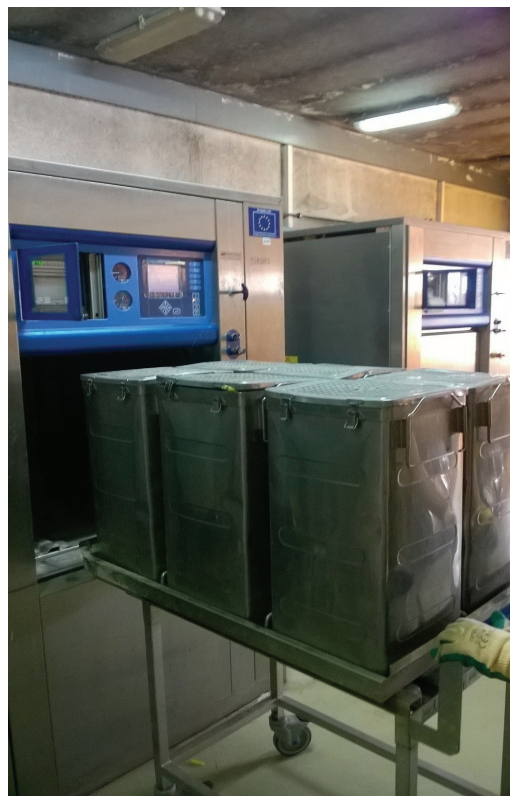
Figure 2. Sterilization of infectious waste in the central waste treatment facility (“CTM”) in the City Hospital in Niš
