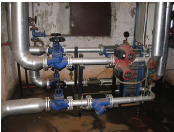
Figure 1. The appearance of the substation installation at 3 Romanijska Street, Niš
